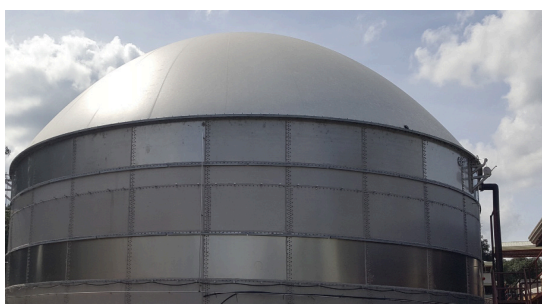
Tank Mounted Storage
