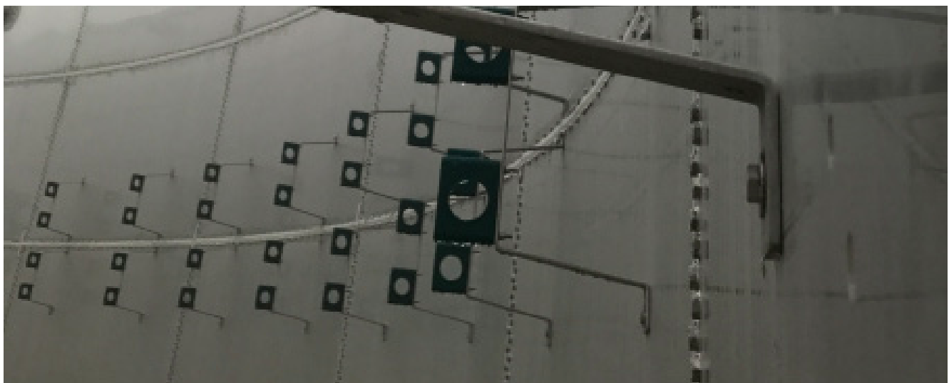
Tank insulation, internal heating, flanges and other fittings.
