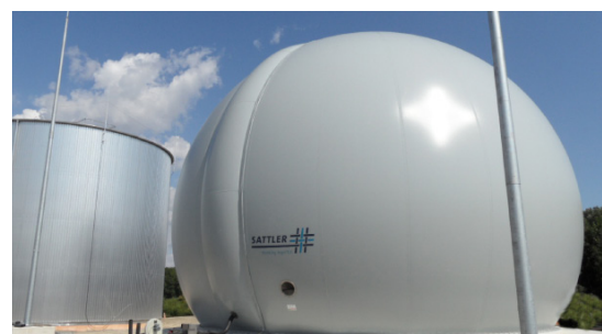
Concrete Mounted Storage
