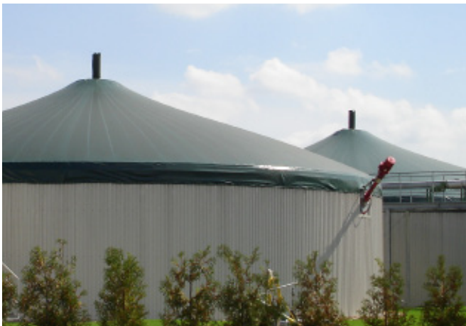
Steel tank mounted
